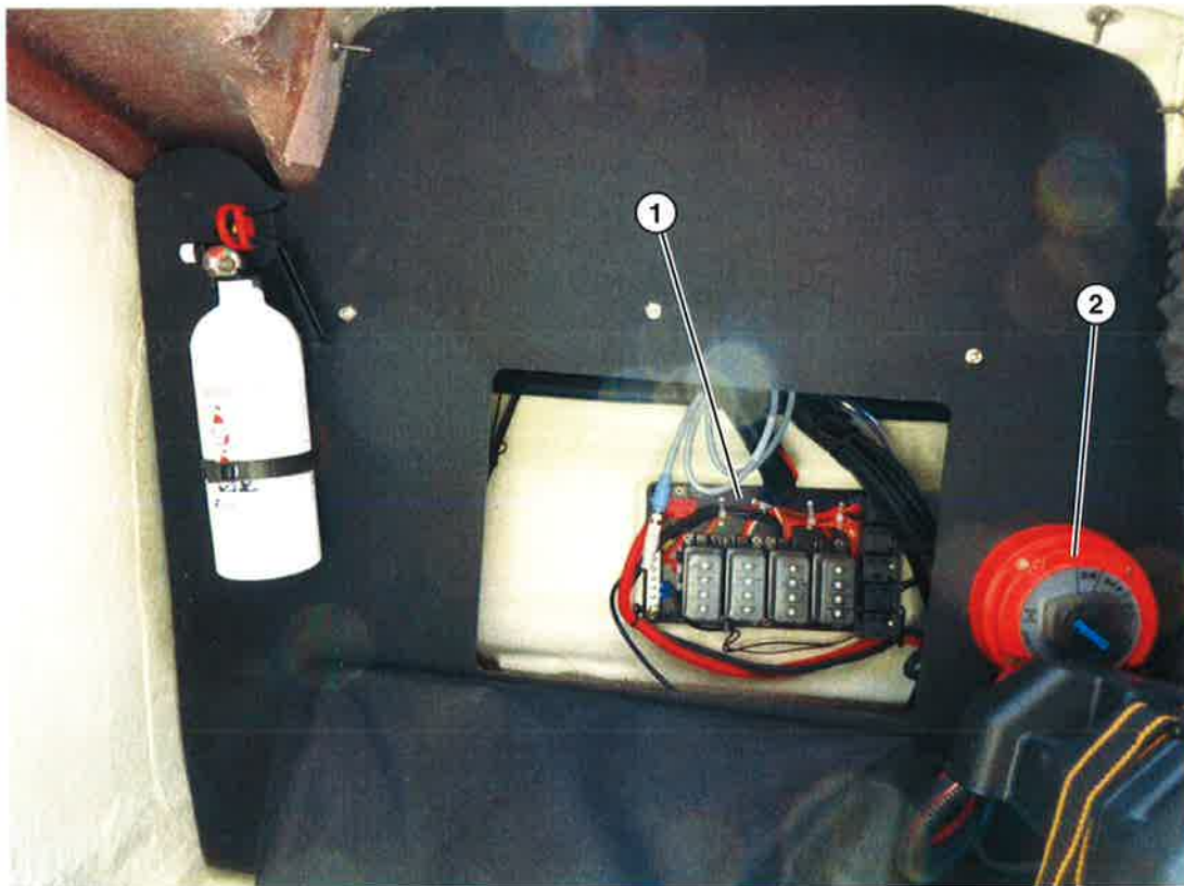
1 – Circuit Breaker Panel
