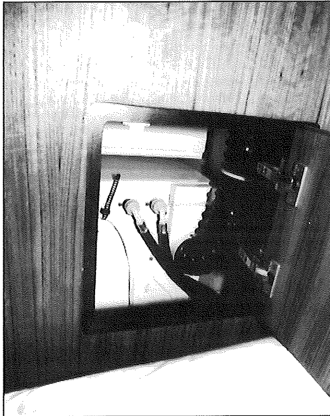
Dryer Lint Trap Access
